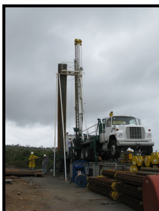
West Indies Power Company drilling rig begins exploratory drilling on the island of Nevis. (Photo: OAS)
