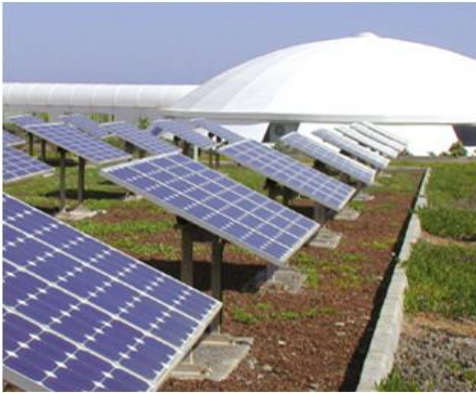
SOLAR PANELS, SOLOMON ISLANDS
